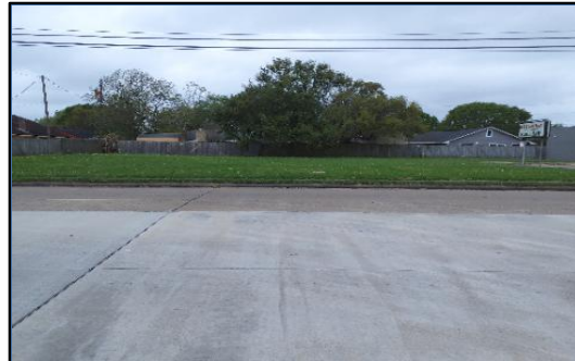
Corner 4 No Ramp (4z)
