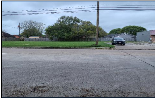
Corner 1 No Ramp (1z)
