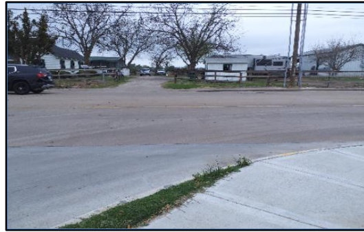
Corner 1 No Ramp (1z)
