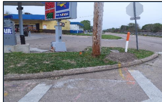
Corner 4 No Ramp (4z)
